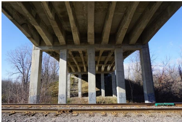
Figure 5: Typical condition of Site No. 27-50 from below
