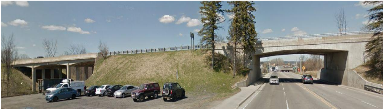
Figure 2: View of the Hawkesbury Creek and CNR Overhead (Left) and County Road 17 Underpass (Right) – Looking North
