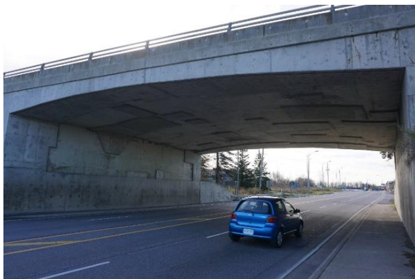
Figure 7: Typical condition of Site No. 27-51 from below
