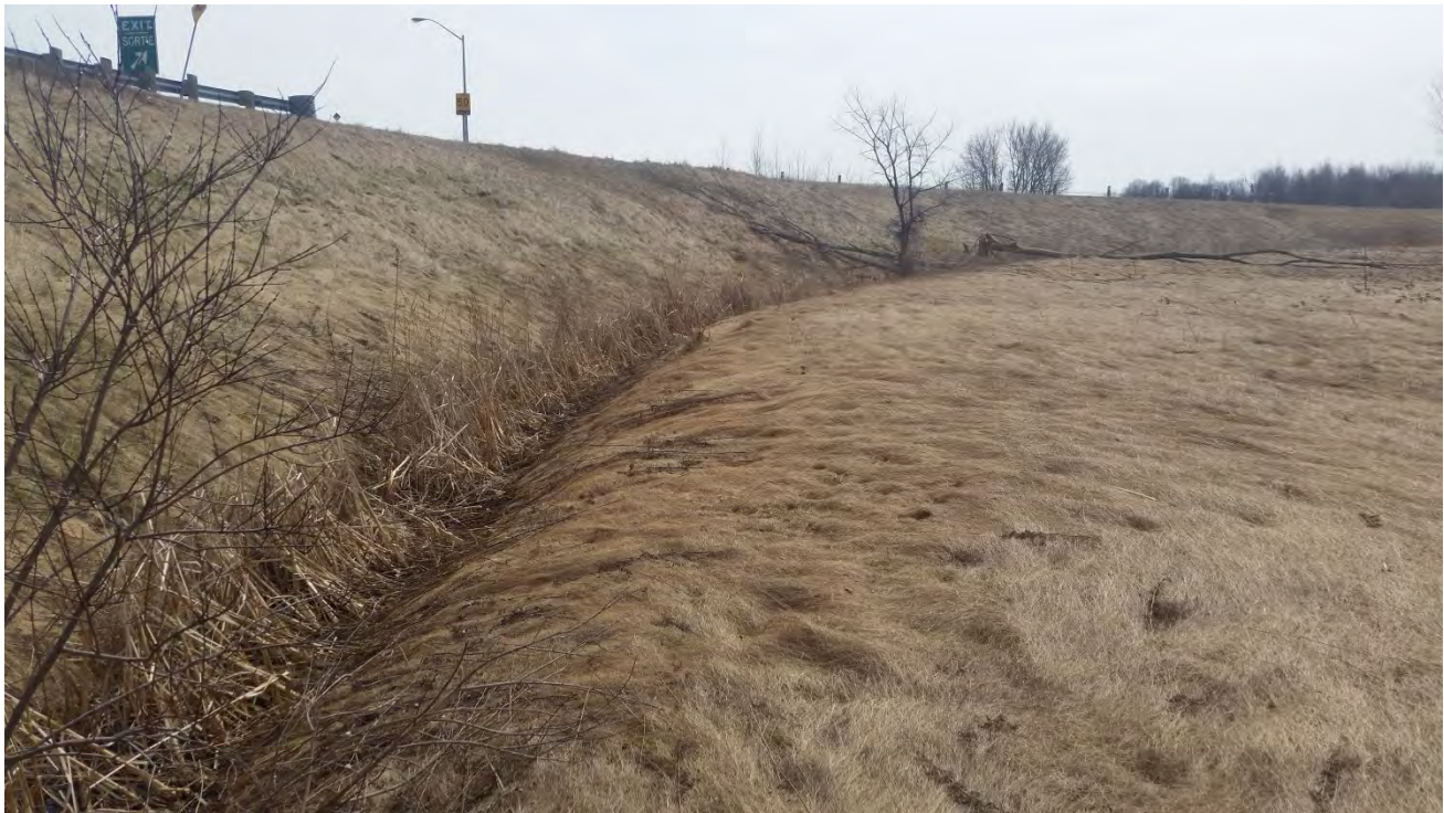
Image 5: Embankment and ditch bordering along the edge of the southeast quadrant facing north.
