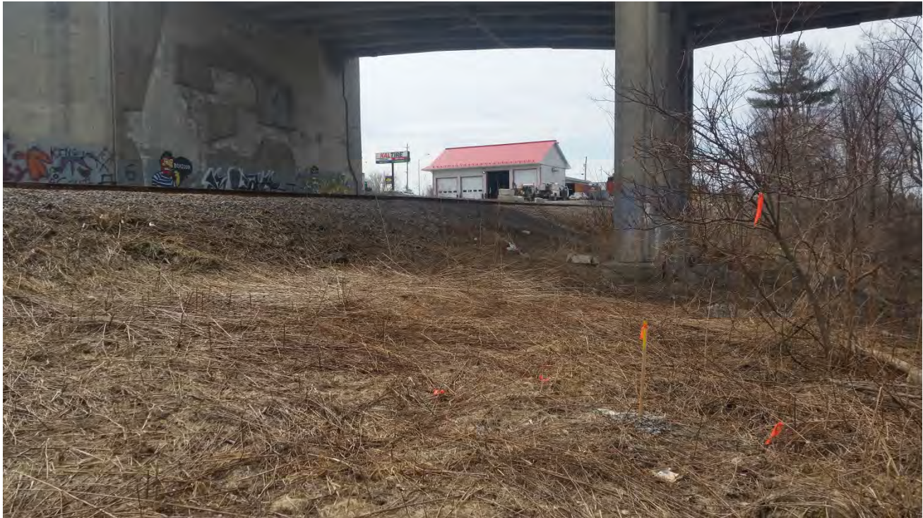
Image 15: Bridge overpass Highway 17 over train tracks in north west quadrant facing south east.
